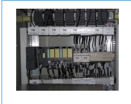
■ Automatons situated in the Ground DOF1 cabinet
