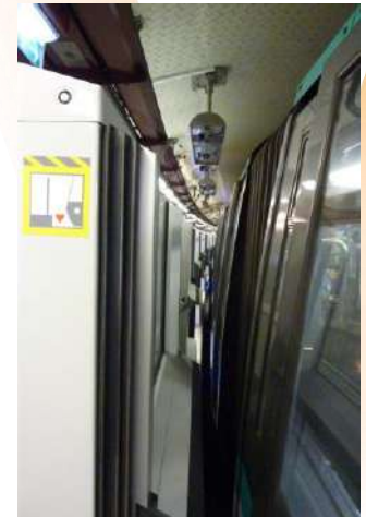
Laser sensors monitoring gaps
