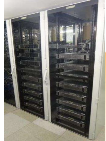
RBC Test Bench hardware installed in a cabinet together with tested equipment
