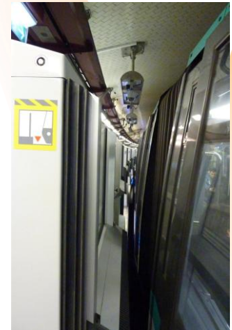
Laser sensors monitoring gaps
